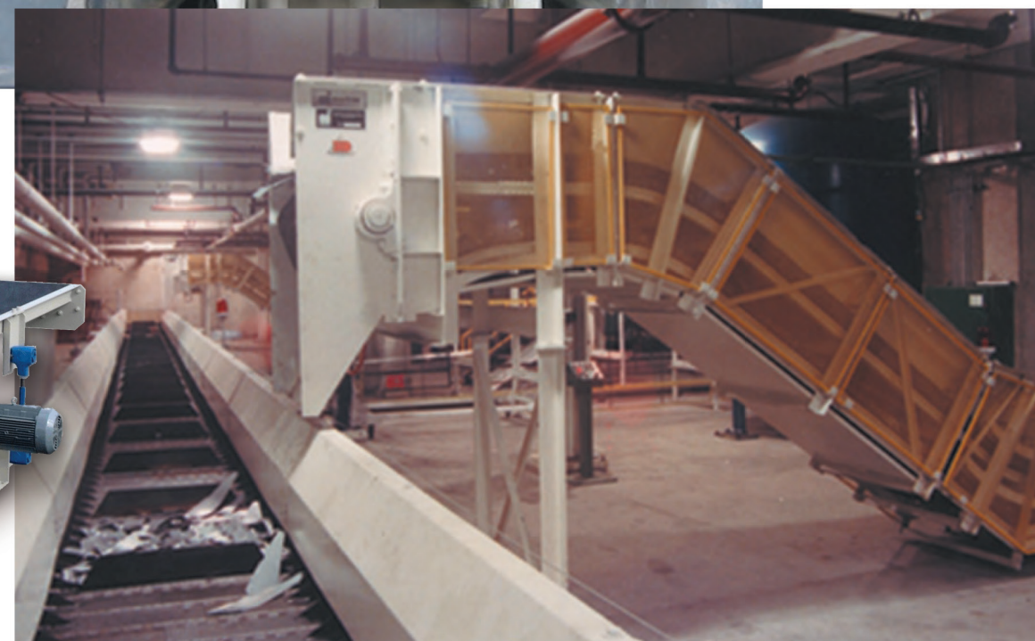
Collector conveyors move scrap from the presses discharging it onto conveyors for elevation to distribution systems.
